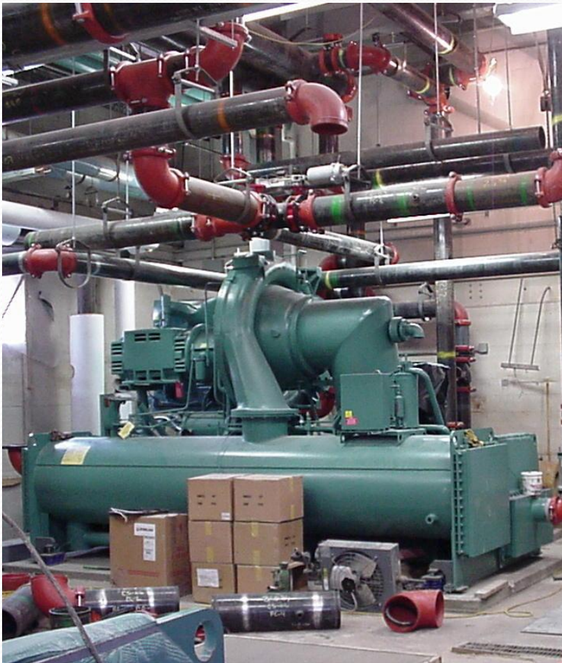
Compression refrigerating machines (CHM)
