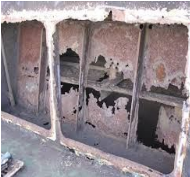
Inoperable fire damper. Wastage found after removing cover.
