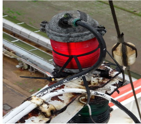
Signal lights not properly secured
