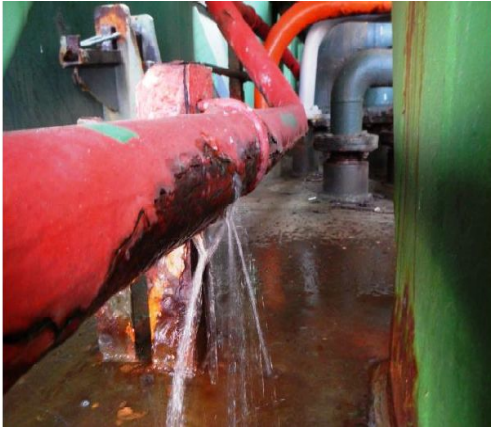
Leaking fire line
