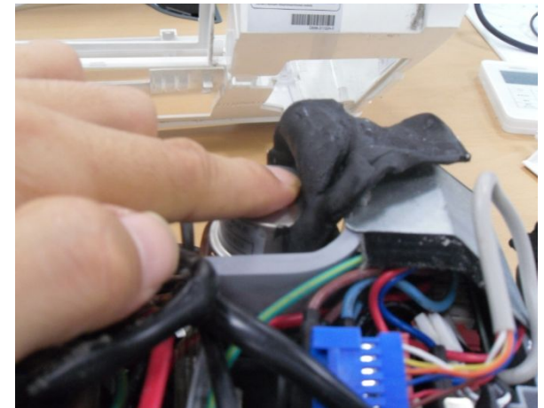
Check operation EEV
