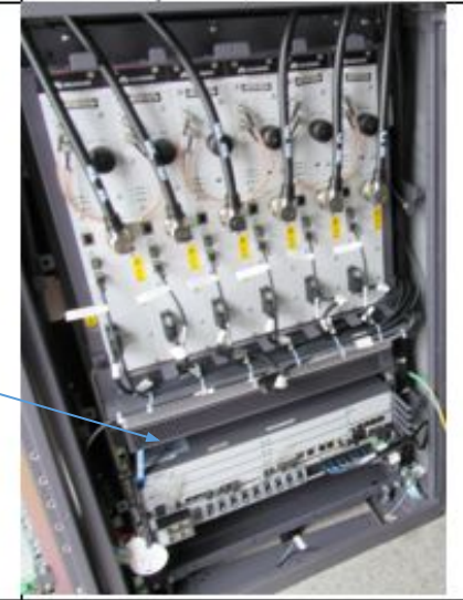
фото BTS, Rack 19" Front view - 2
