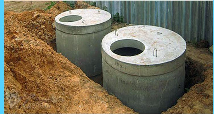
6. Tanks for TUZ drainage.
