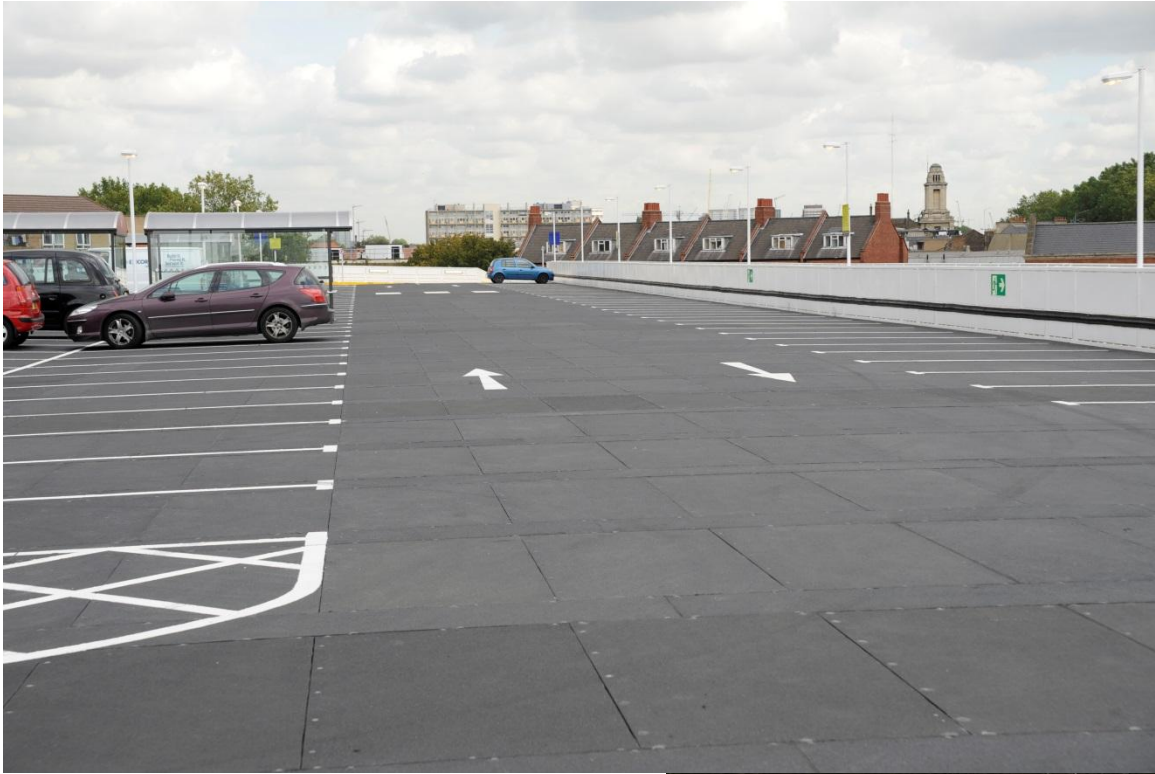
Gen 1 – 3 Panels Water drained through panels to RL60 then to gutter box on column line
