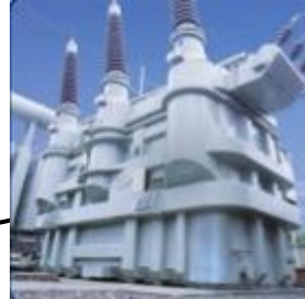
Step up transformer
