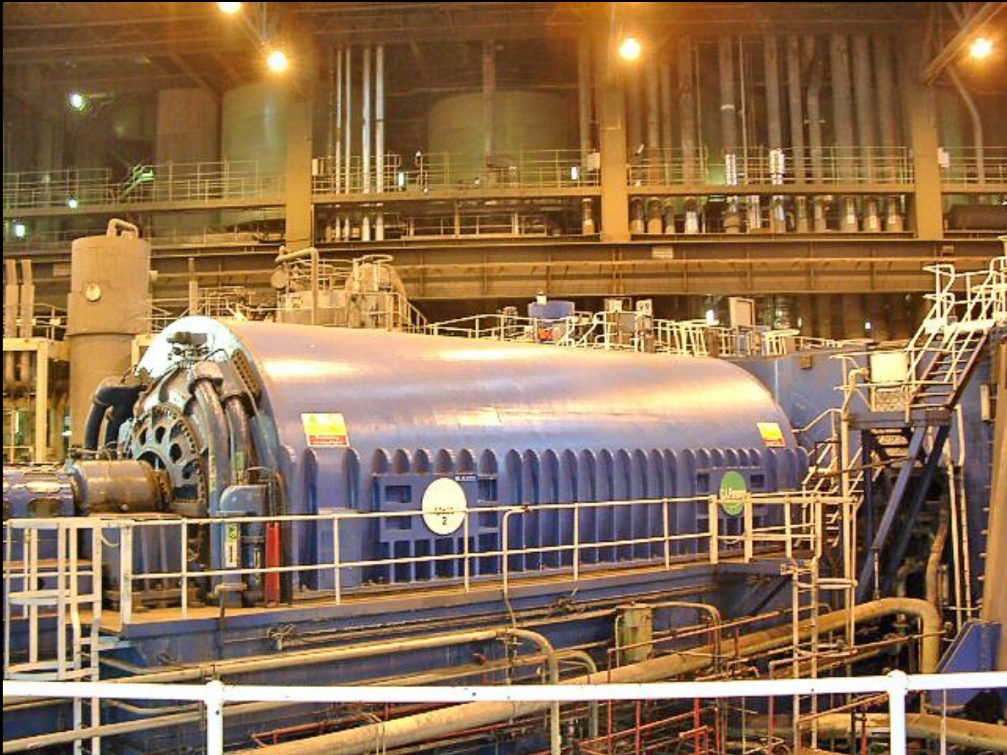
A generator at Drax power station in England
