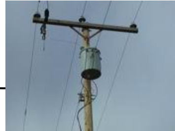
Step down transformer
