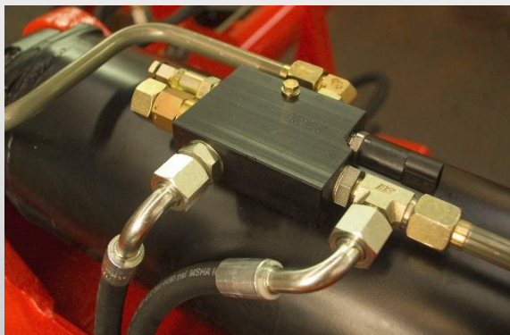
Block valve on the lifting rams
