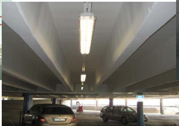
Low bay lighting
