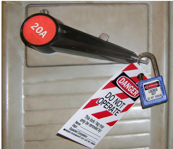
MAIN SWITCH LOCKED OUT
