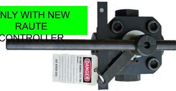
DISCHARGE VALVE CLOSED AND LOCKED OUT
