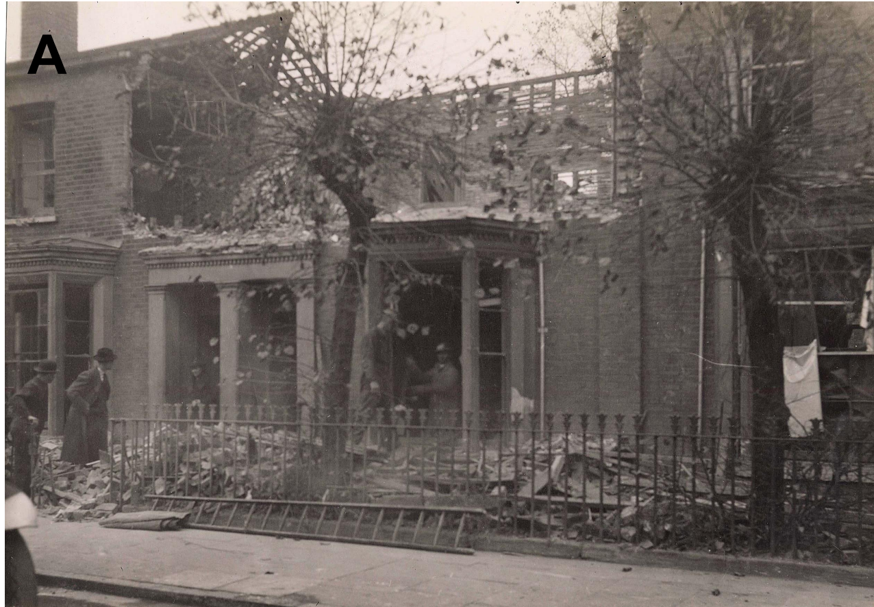
Bomb damage to 103 Mapledene Road, Hackney, following an attack by the German Air Force with high explosive bombs on 21/22 October 1940.
