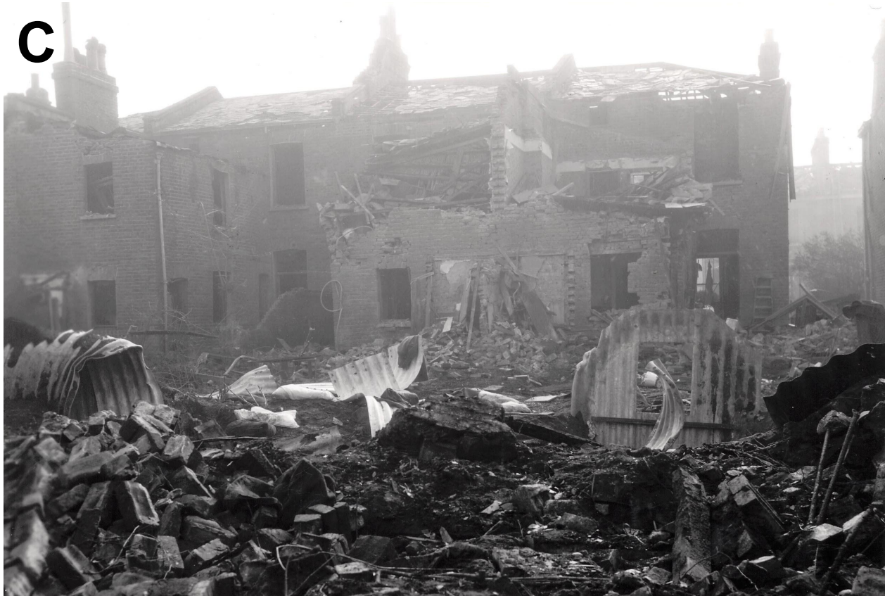
Bomb damage to 127-129 Mapledene Road, Hackney, showing damage to rear of houses and gardens, following an attack by the German Air Force with high explosive bombs on 09/10 October 1940.
