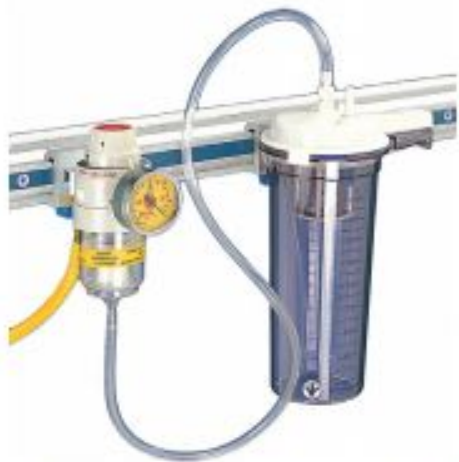
Functioning suction facilities
