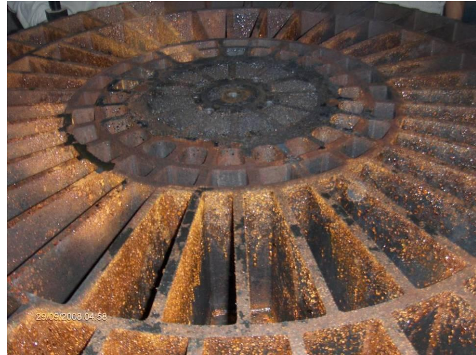
rusty cellular wheel
