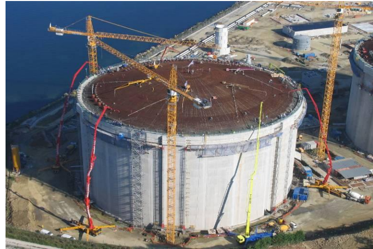
LPG tank, Spain
