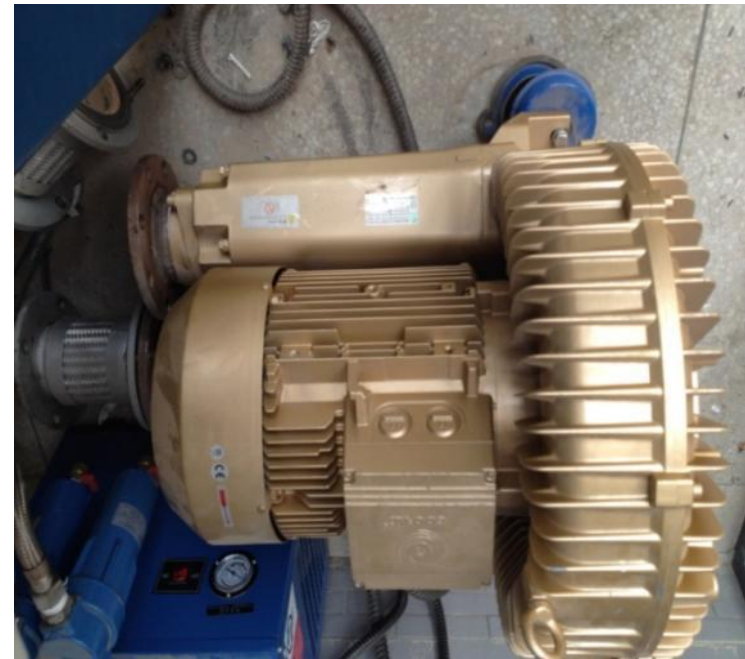
Central waste suction machine
