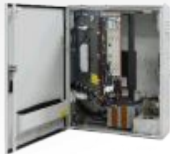
In Outdoor Cabinet
