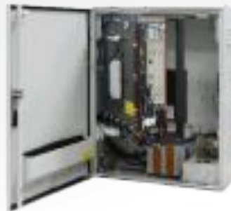
In Outdoor Cabinet
