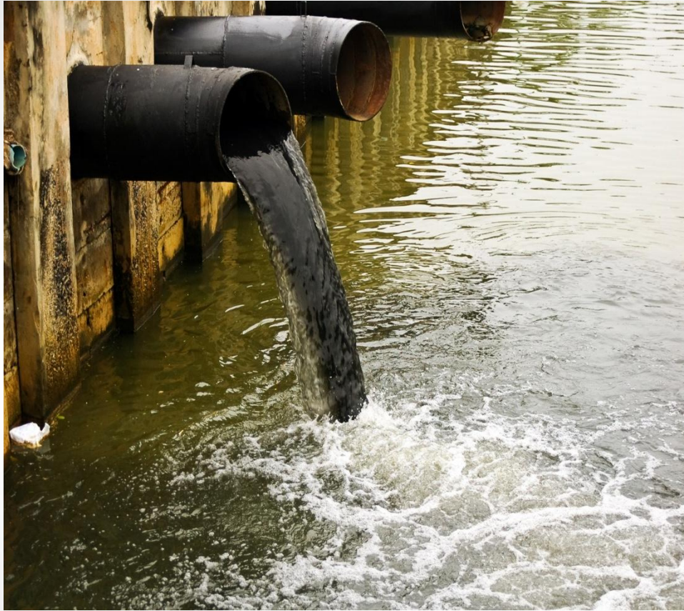
Drain pipes in France
