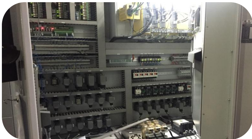
Three-door electric cabinet, reasonable electrical components layout
