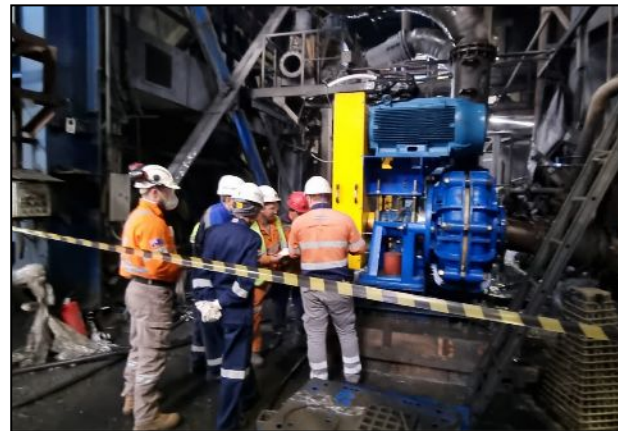
RHS – Pump 56, 66 & 67 C1 checks
