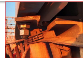
Tube bundle #93 support #1 damage
