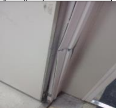
Damage to BARS metal door frames from propelled air cylinder
