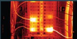
Circuit Breaker Problems
